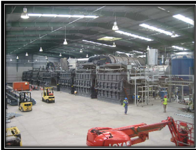
Scotgen facility near Dumfries, Scotland
